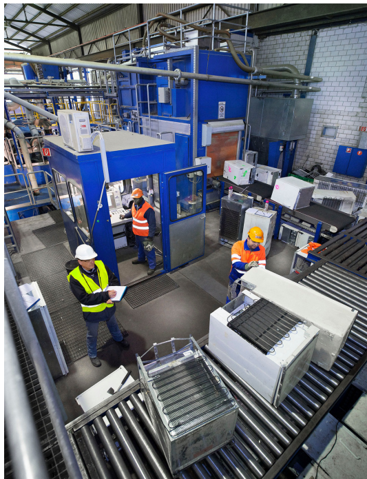
A look into a refrigerator treatment system
